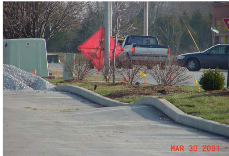
Fluid pressure causes damage to surface areas
