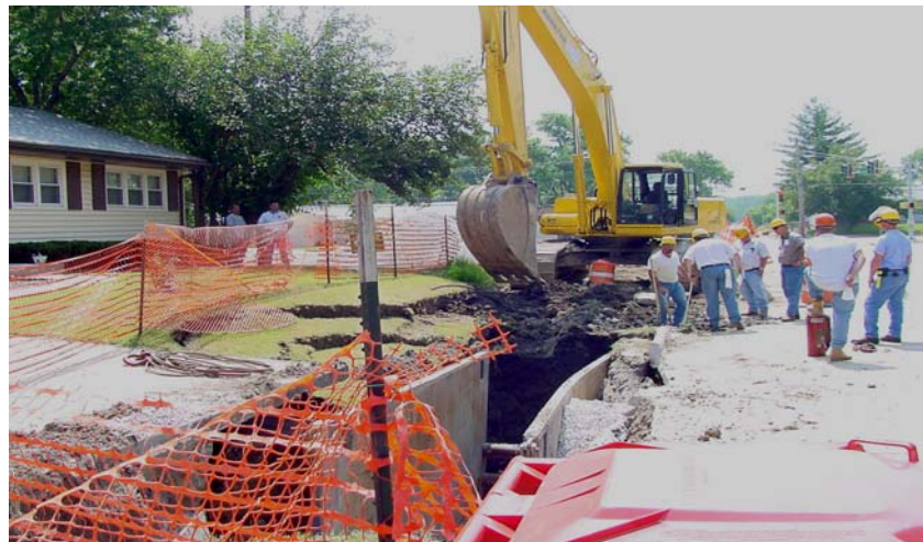
Open trench methods cause damage to surface areas
